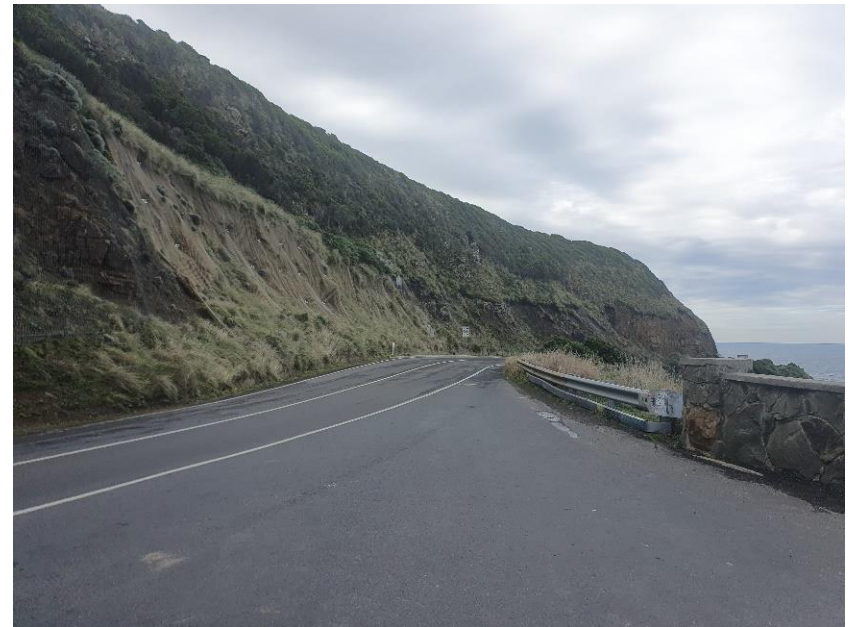
Example of rock bolting employed along a section of Great Ocean Road (photo taken by T+T)
