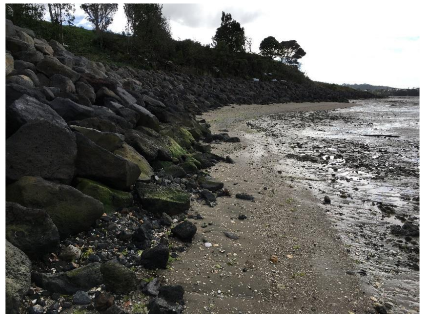
Rock revetment protecting cliff toe in Auckland, New Zealand (Photo taken by T+T)
