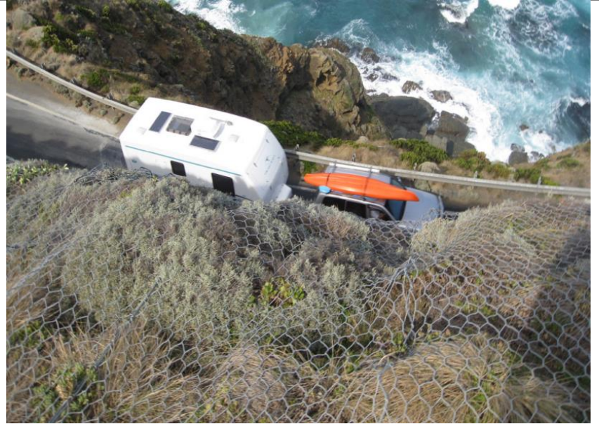
Source: Great Ocean Road rockfall protection. CaseStudy_Steelgrid_GreatOceanRoad2009.pdf (rockfall.co)
