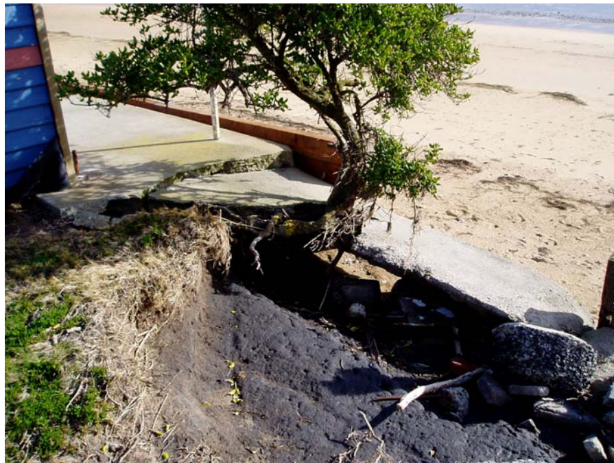
Erosion adjacent to a beach shack.
