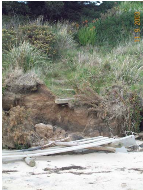
Eroded access steps at the base of Jam Jerrup cliff
