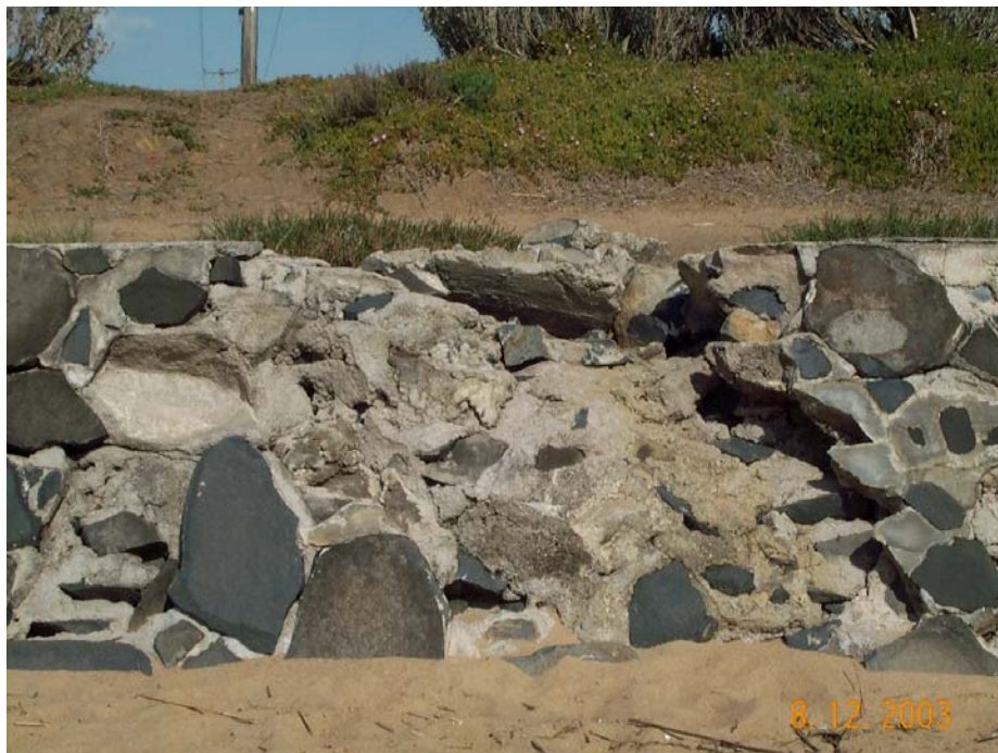
Erosion of the seawall close to Lang Lang Jetty
